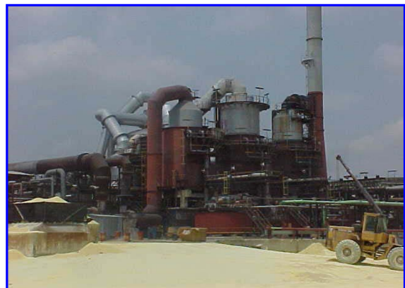
No 4 Sulphuric Acid Plant at Sasol Agri Phalaborwa
