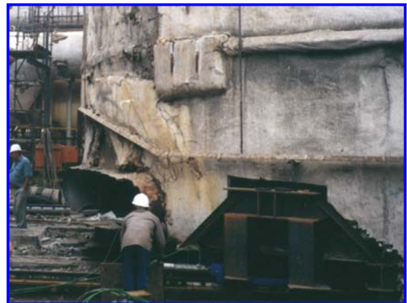
Old Converter sliding off foundation
