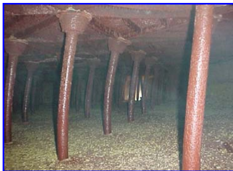
Bent posts in lower Converter pass
