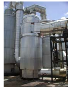
All stainless Reheat Exchanger installed at Sasol Agri., (South Africa) July 2002 during phase 2 of acid plant retrofit
