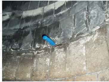
Damaged joints in a venturi
